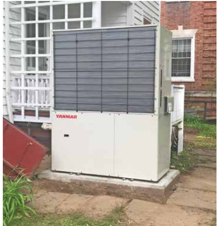
Yanmar's 14-ton gas heat pump VRF system provided a cost-effective heating and cooling solution to help the YMCA of Northern Middlesex County upgrade its HVAC system.
