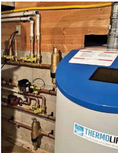
PHOTO COURTESY OF THERMOLIFT INC.
